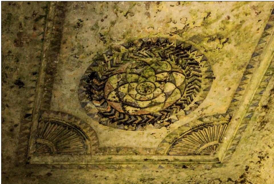
Pic: Ruined roof Designs
